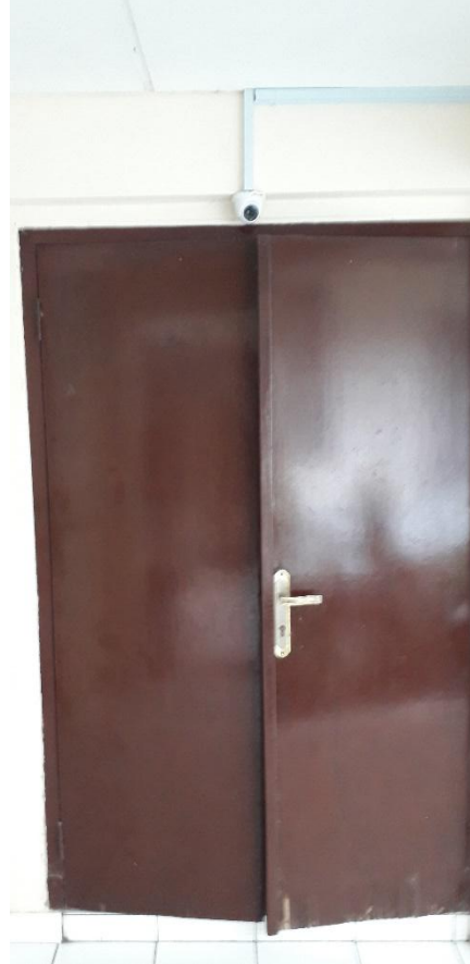
Cctv Area Lorong
